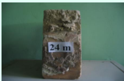
Brick samples from cement kiln at 24m indicated heavy discoloration due to infiltration of gases
